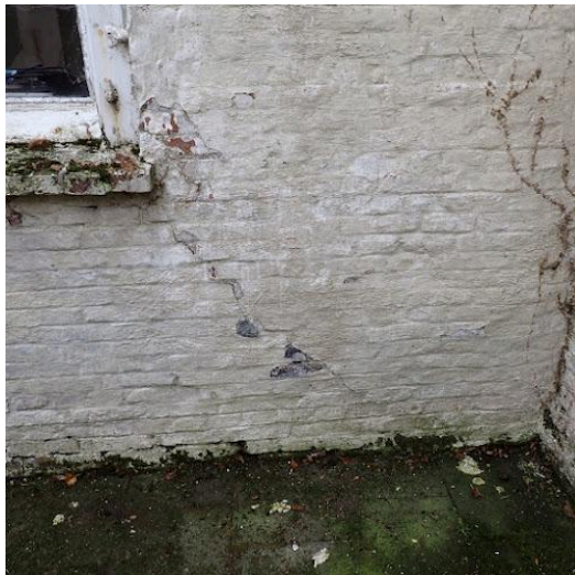
vleugel [3]-west: lichte scheurvorming
