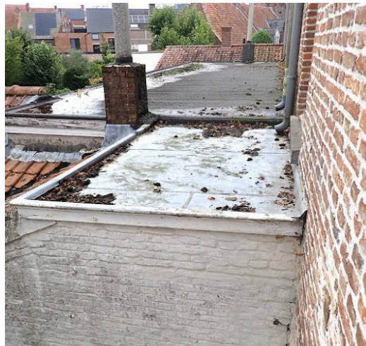
dak [2]: vezelcementen schoorsteenpijp is asbesthoudend
