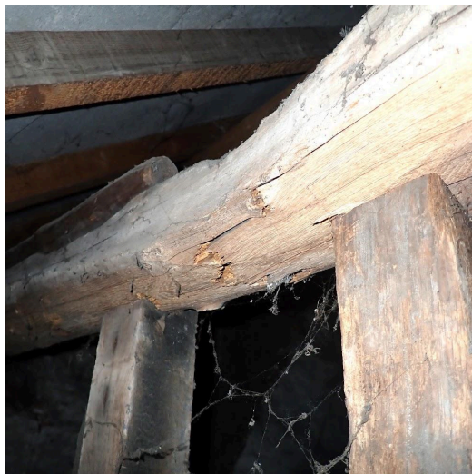
dak [1]: doorgebroken gording
