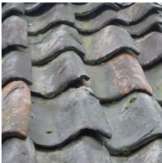
dak [1]: afgebroken pan
