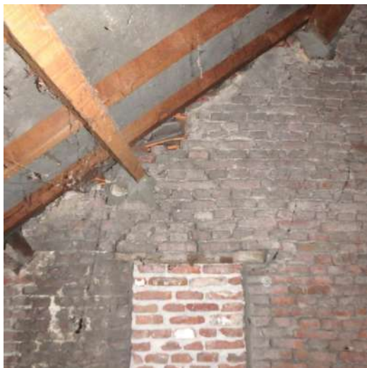
zolder [1]-west: scheurvorming
